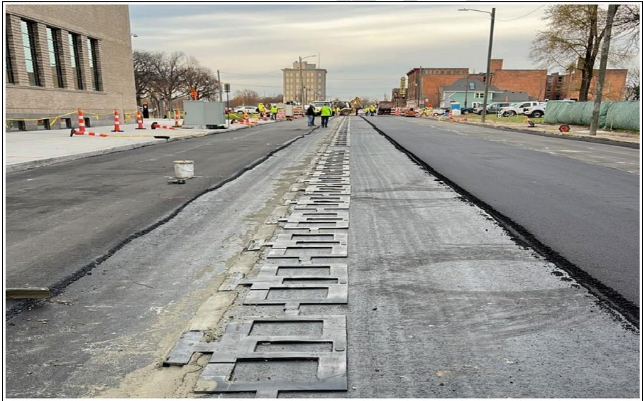
Figure 8: Dynamic Inductive Charging Infrastructure
